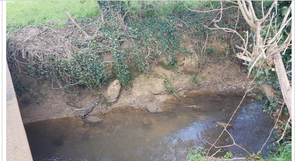
Photo 125: Collapse of bank material on outer meander immediately downstream of bridge
