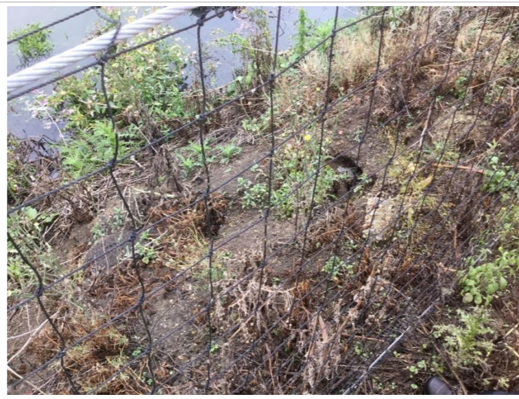
Photo 98: Animal burrowing in failed banks
