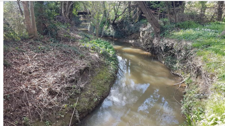
Photo 127: Upstream towards bridge from left bank showing erosion on outer meander bank face and vertical bank profile. Heavily shaded.
