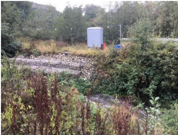
Photo 3: Gabion mattresses and erosion of bank
