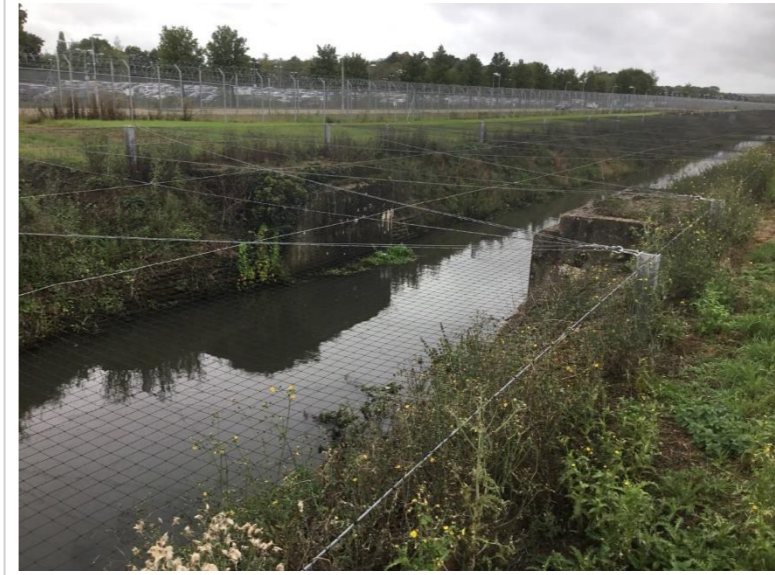
Photo 105: Former bridge abutments and spillway connecting to outfall on left bank at Car Park X
