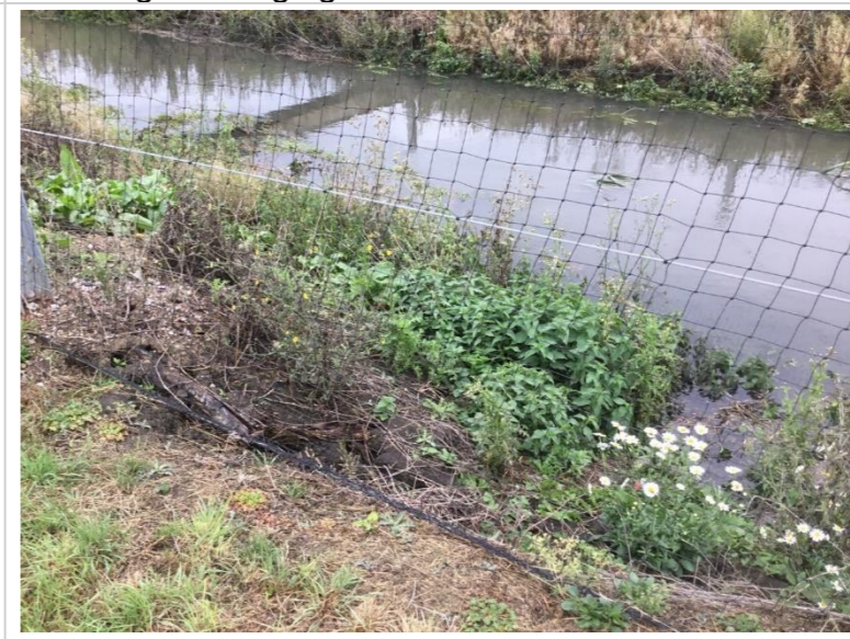
Photo 99: Bank erosion extending under bird netting on right bank
