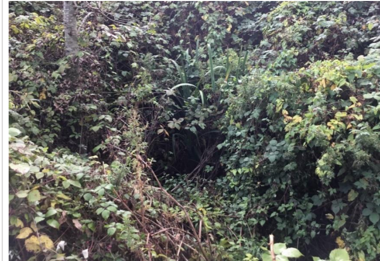
Photo 114: Culvert outlet heavily vegetated
