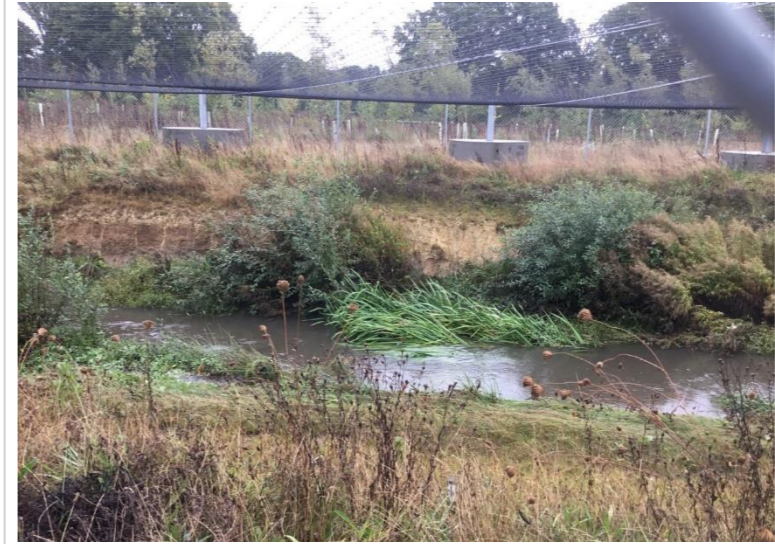
Photo 49: Tall emergent grasses formed along margins of channel, erosion of steep right banks
