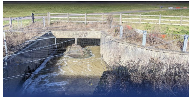
Photo 8: Runway box culvert inlet with debris trapped on divider wall
