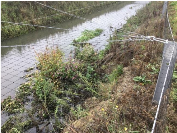
Photo 3: Bank erosion downstream of gabions
